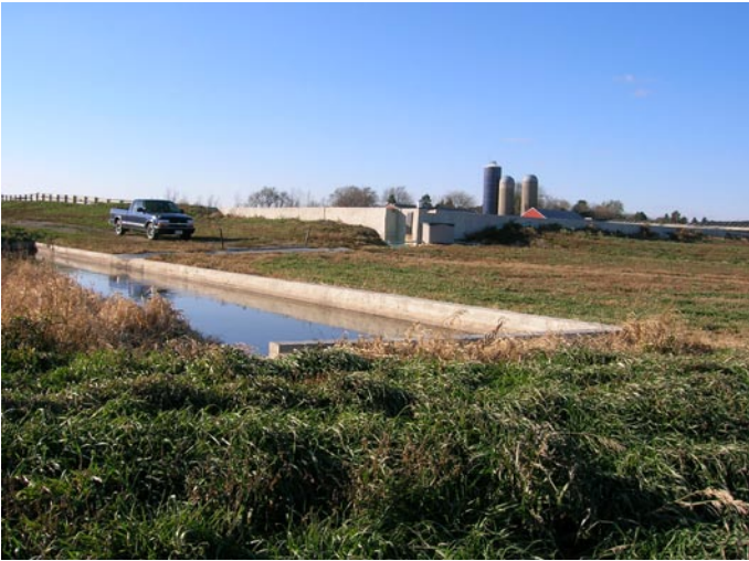
Concrete spreader between SS basin and VTA channel distributes the settled effluent across the entire width of the channel.
